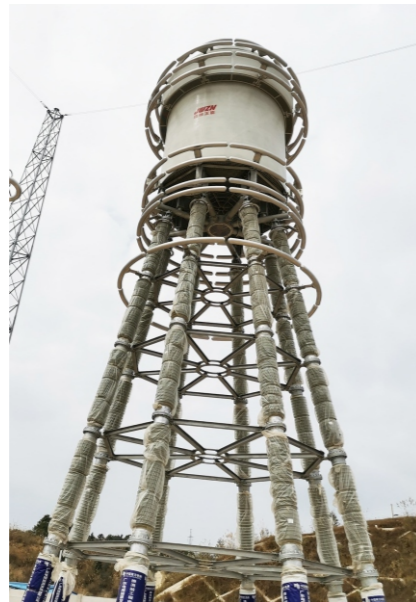
Wudongde ±800 UHVDC Multi-terminal Project 800kV Smoothing Reactor-HV
