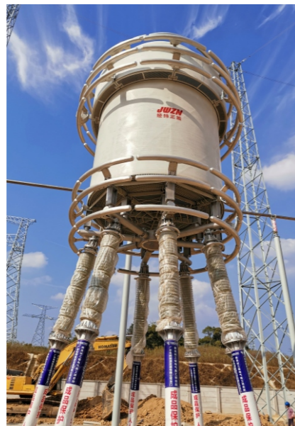
Wudongde ±800 UHVDC Multi-terminal Project 800kV Smoothing Reactor-LV
