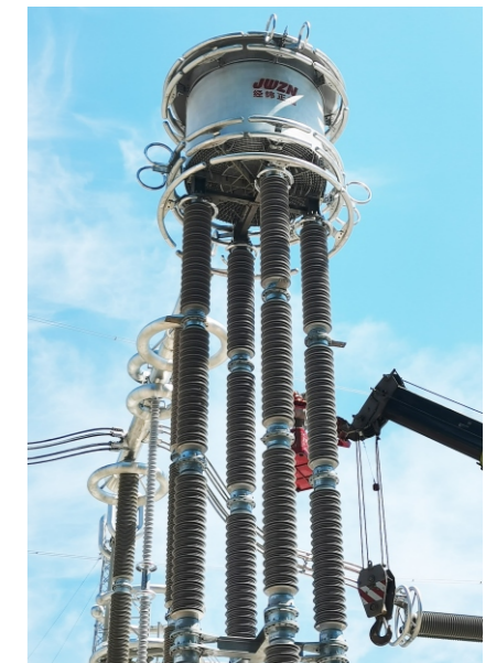
Shaanxi North - Wuhan ±800 kV UHV DC transmission project PLC Reactor
