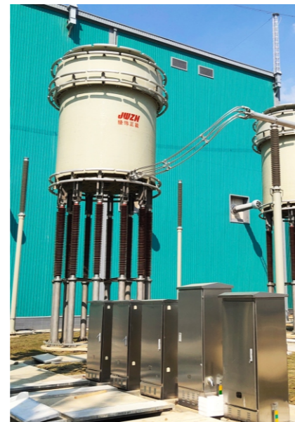
Baihetan - Jiangsu ±800 kV UHV DC project 215kV Converter Reactor-LV
