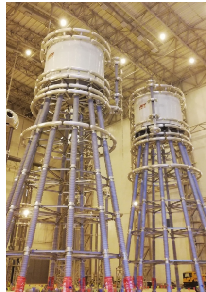
Changji-Guquan ±1100kV UHVDC 1100kV Smoothing Reactor -HV
