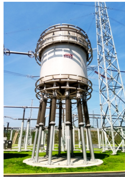
Changji-Guquan ±1100kV UHVDC 1100kV Smoothing Reactor-LV
