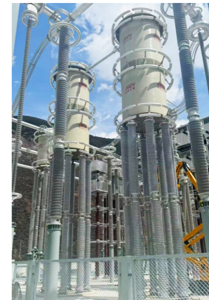
Jinshang-Hubei ±800 kV UHV DC transmission project DC Filter reactor
