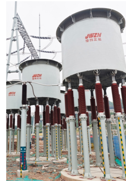
Sichuan-Chongqing 1000kV AC UHV project 110kV Shunt Reactor
