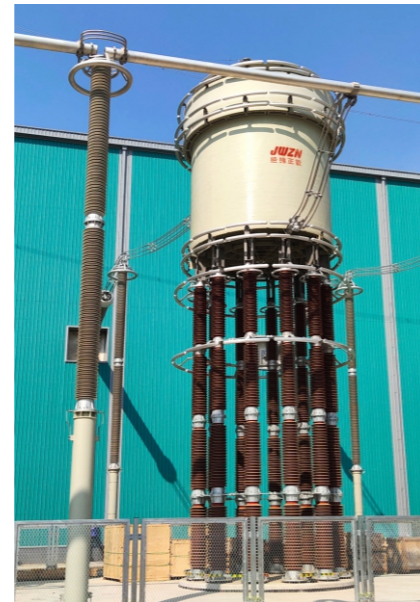
Baihetan - Jiangsu ±800 kV UHV DC project 545kV Converter Reactor-HV
