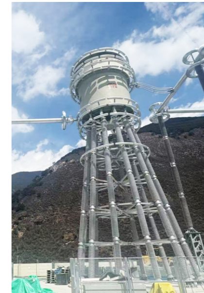
Jinshang-Hubei ±800 kV UHV DC transmission project 800kV Smoothing Reactor
