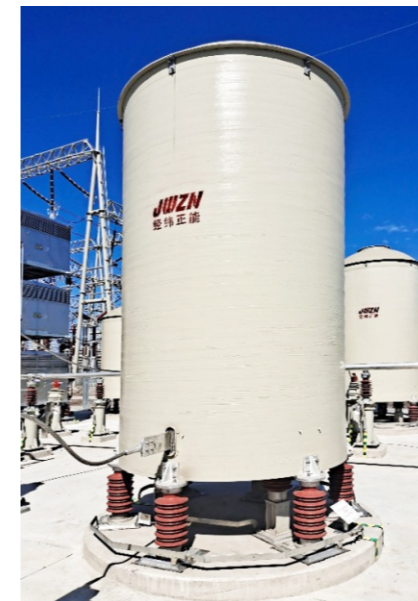
Zhebei ±800kV HVDC 110kV Filter Reactor
