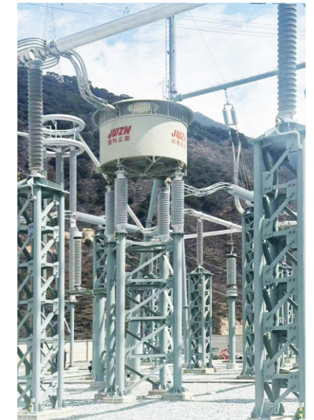
Jinshang-Hubei ±800 kV UHV DC transmission project TDR Reactor
