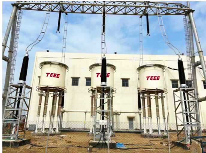
900MW Combined Cycle Power Station in Pakistan 220kV Current Limiting Reactor
