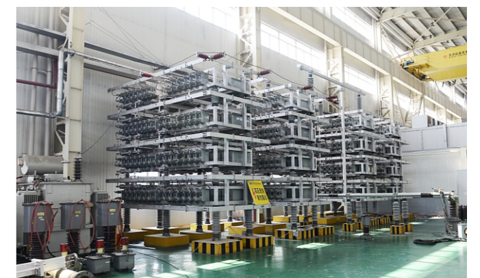
Capacitor Banks (up to 60kV) for AC Temperature Rise Testing
