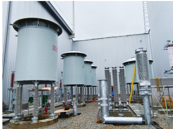
CATL Xiapu Project Converter Reactor, 1220A
