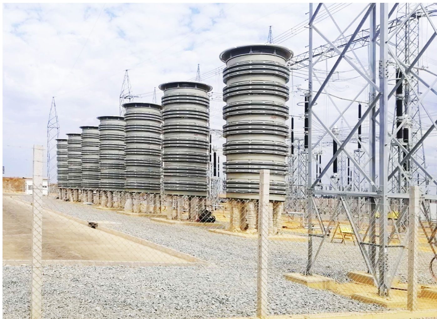
SILVÂNIA Substation Project in Brazil 500kV Shunt reactor
