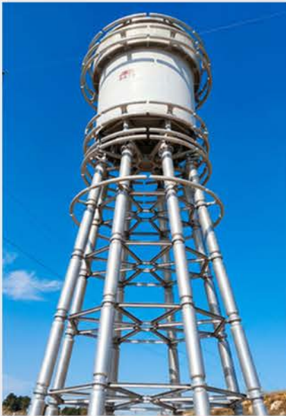
Wudongde ±800 UHVDC Multi-terminal Project 800kV Smoothing Reactor-HV
