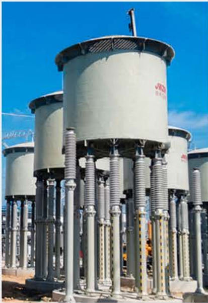
Jingmen 1000kV UHVAC 110kV Shunt Reactor
