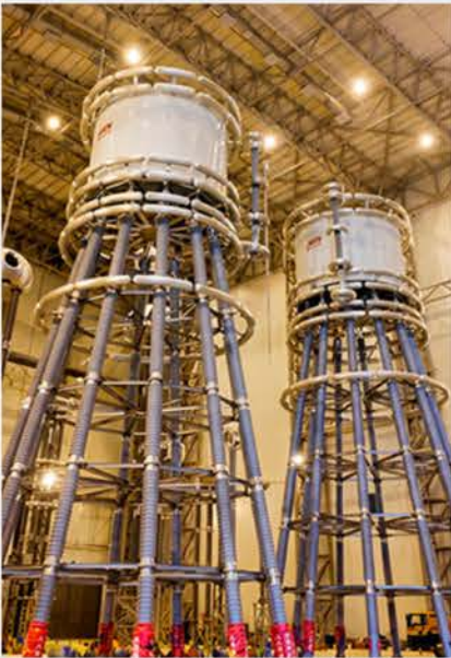
Changji-Guquan ±1100kV UHVDC 1100kV Smoothing Reactor -HV
