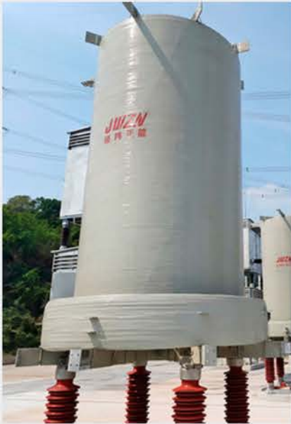
Zhebei ±800kV HVDC 110kV Filter Reactor
