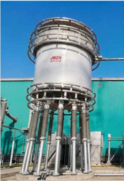
Changji-Guquan ±1100kV UHVDC 1100kV Smoothing Reactor-LV
