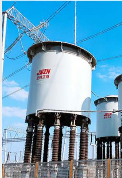
Jinzhong 1000kV Substation Project 110kV Series Reactor
