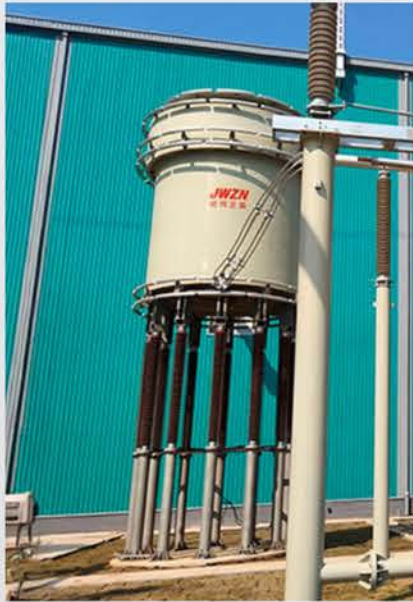
Baihetan - Jiangsu ±800 kV UHVDC project 500kV Converter Reactor-HV
