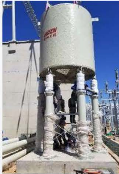
Changtai Substation 110kV Shunt Reactor
