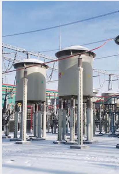
Zhangbei 500kV VSC 66kV Shunt Reactor
