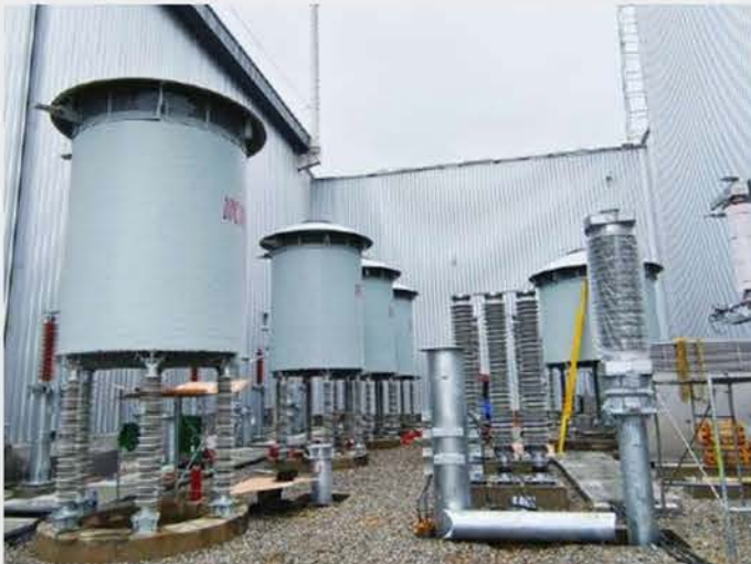
CATL Xiapu Project Converter Reactor, 1220A
