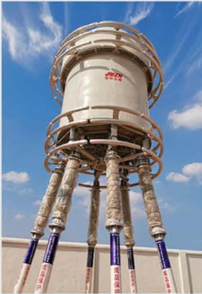
Wudongde ±800 UHVDC Multi-terminal Project 800kV Smoothing Reactor-LV
