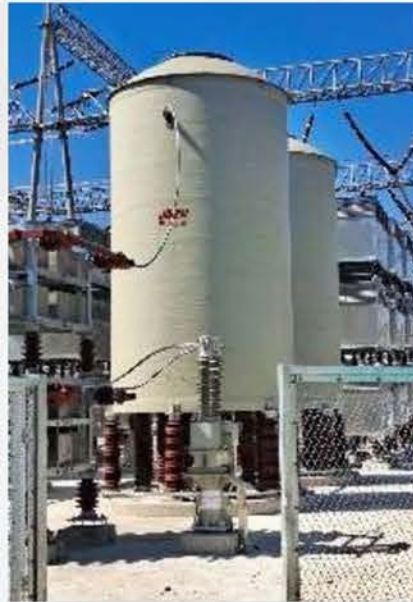
Zhangbei-Shengli 1000kV HVAC 110kV Series Reactor
